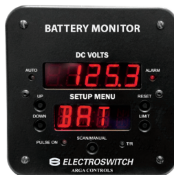
Substation Battery Monitor
